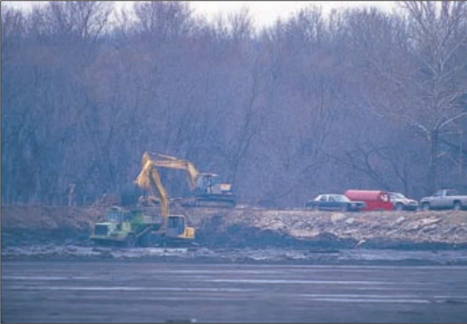
The Marais des Cygnes River eroded its way close to the Miami State Fishing Lake dike. Borrow to rebuild and fortify the dike was taken from the lake bed, reducing the project's impact on the surrounding area and creating better fish structure.
